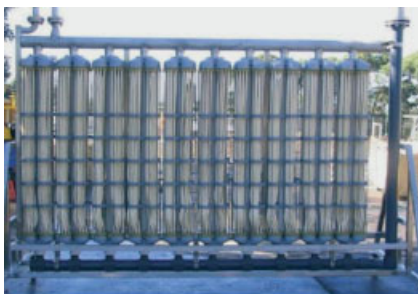
D: HF/CT membranes mounted in frame
